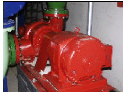
Bell & Gossett equipment was chosen for the cooling system upgrade to Brazil's central bank because of energy and space efficiency.
