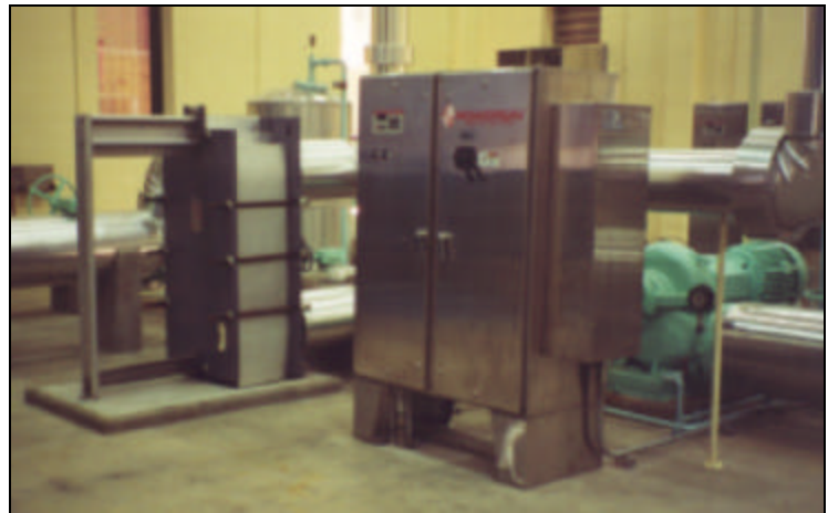
Inside the plant, pumps and control systems from Bell & Gossett work to keep anaerobic bacteria at just the optimum temperature.
