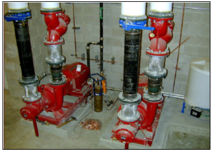
Behind the scene, Bell & Gossett pumps, heat exchangers and control systems are found throughout the new stadium's H.V.A.C. and water supply system.
